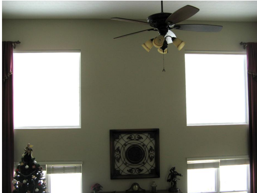
B. Photograph indicates area in which above thermogram was recorded - Great Room, north elevation.
