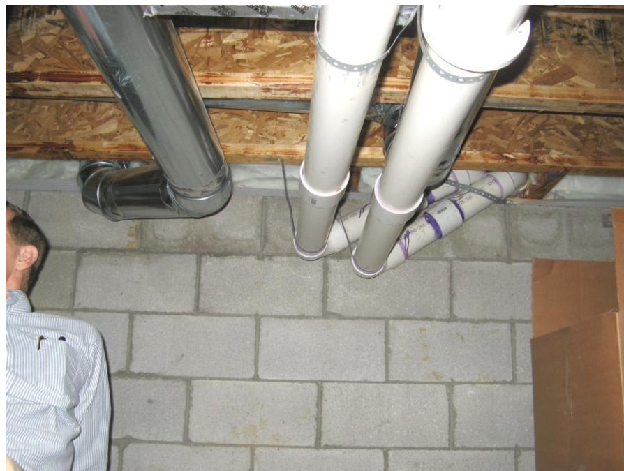
B. Photograph indicates area in which above thermogram was recorded - Basement, west wall.
