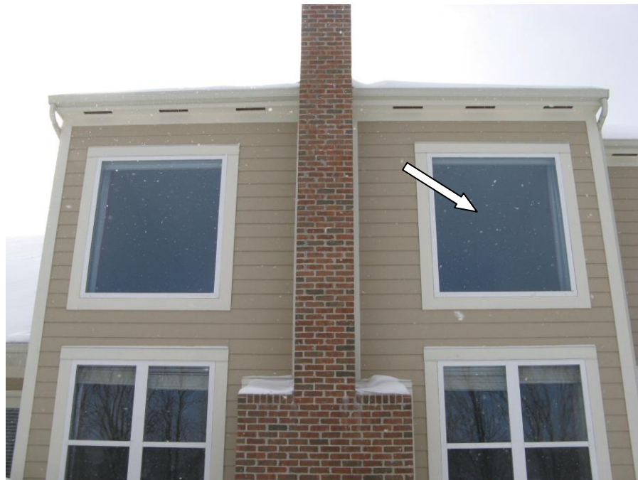
B. Photograph indicates area in which above thermogram was recorded - exterior, north elevation.
