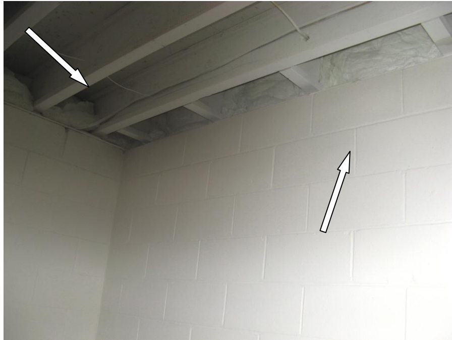
B. Photograph indicates area in which above thermogram was recorded - Basement, east wall.
